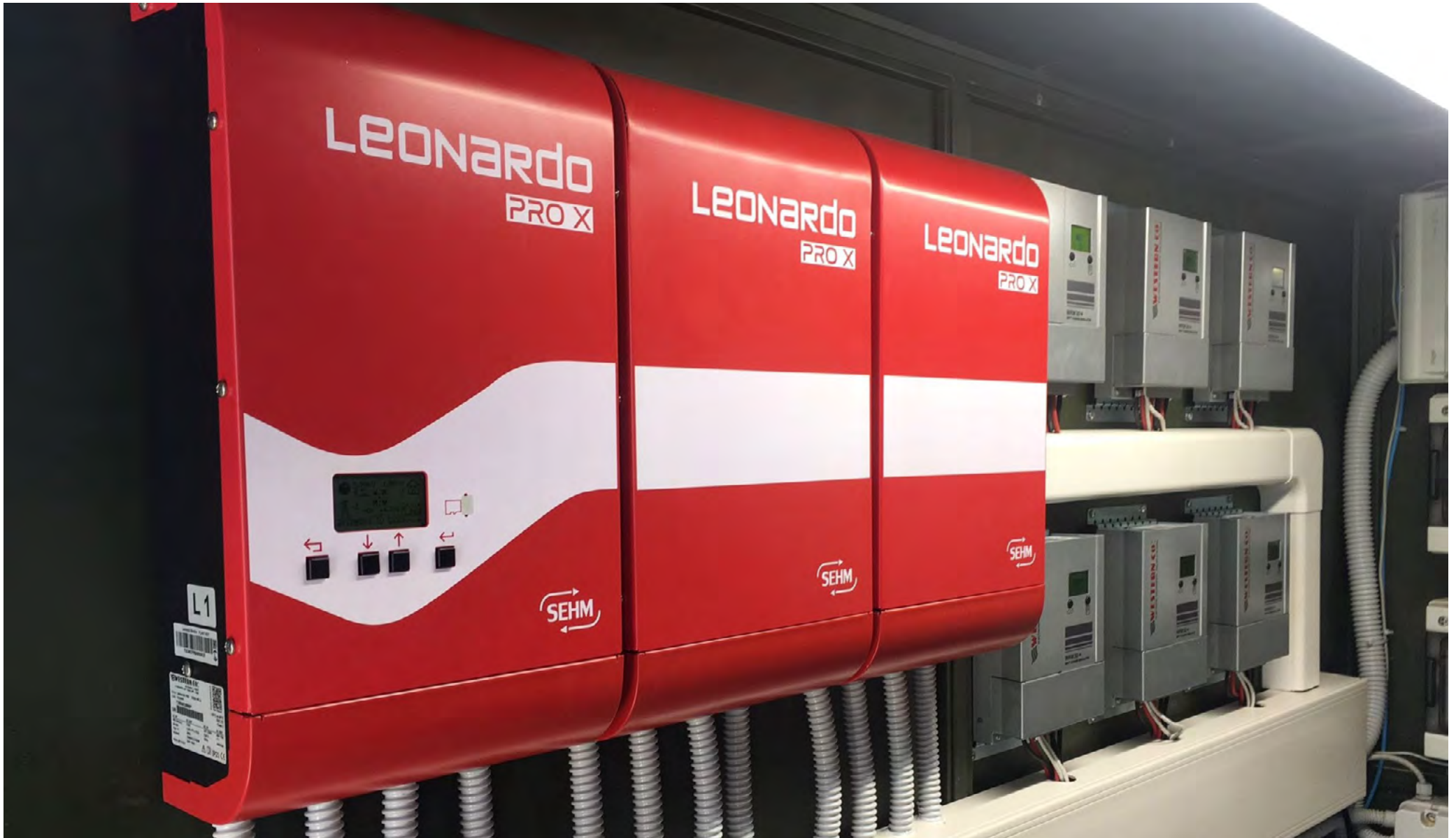
Leonardo PRO X - Triphase Pylontech Terni - Italy
